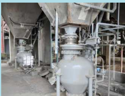
ESH System for handling Ash
